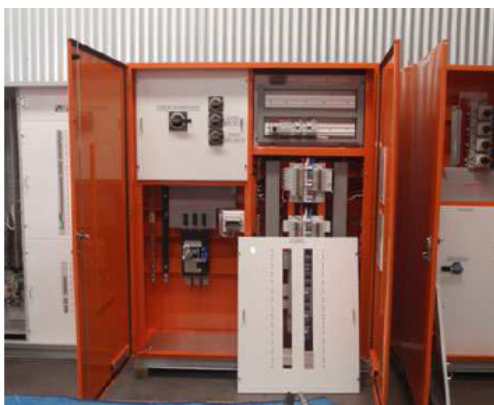
Mechanical Services Switchboard
