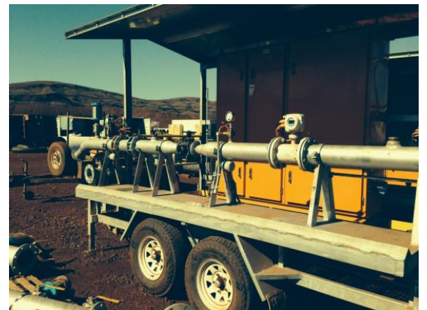
Trailer Mounted Bore Pump Starter/Control Panel
